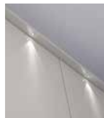
Built - in lighting
